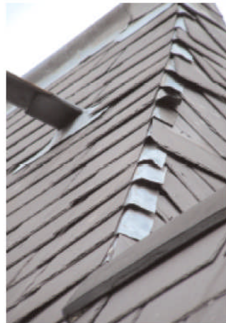
This is what lead soakers look like on a mitred hip, when the cut slates on one side have been blown off because they were only once nailed
