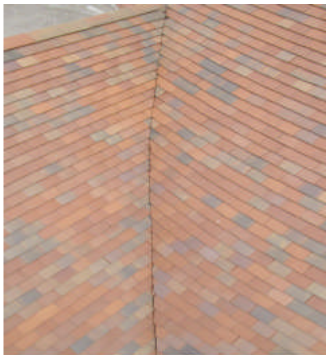
The straight section of roof is on the left and the conical roof is on the right. Note how the valley bends to the right. It is a shame that the valley has been incorrectly detailed as a secret valley as it will cause problems in the near future
