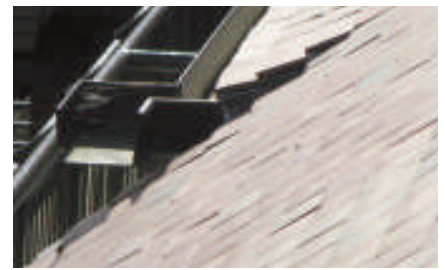
The clay plain tiles have been formed into a sprocket over an inset balcony. The sprocket diminishes to nothing over four courses. With a steeper pitch it may be over five courses
