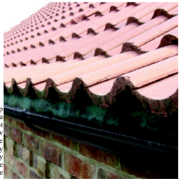
The difference in true tile pitch between the first and second course may not look very much but is more than 5°. This was caused by the brick corbel eaves detail being one brick too high. This is not helped by the guttering being too low
