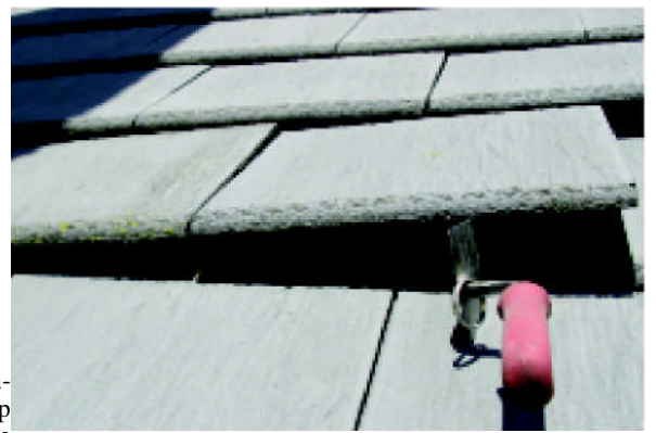
Light weight concrete interlocking tiles should always be head nailed and tail clipped, unlike these tiles that were chattering in the wind
