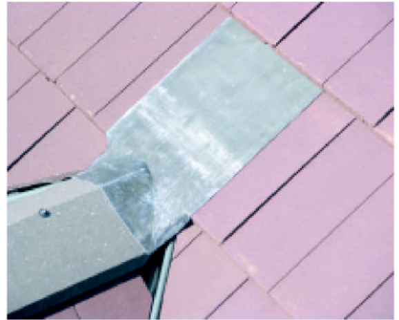
The 300mm-wide lead saddle does not lap the ridge tile by 150mm at the edges, is not clipped down against high winds, and does not lap the GRP dry valey below by 250mm (true valley pitch 17.5°). But otherwise is quite neat!
