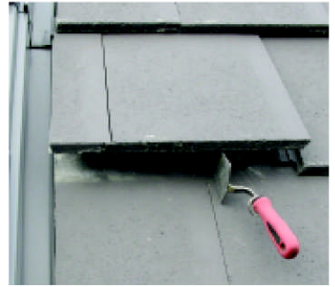
Every tile on this roof should have been twice nailed and once clipped. Clearly the verge clips were missing.
