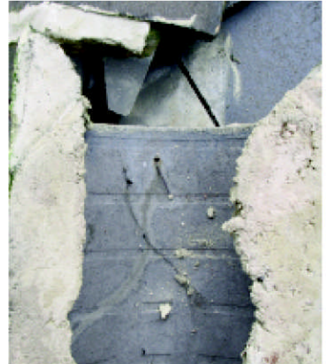
Whilst there is plenty of mortar on the underside of this hip tile, none of it adhered to the roof tiles. There was no mortar under the end where the nail hole is. Note the ungalvanised steel nail has rusted away and was not fixed into anything, just bent under to look like it was holding the hip tile down.
