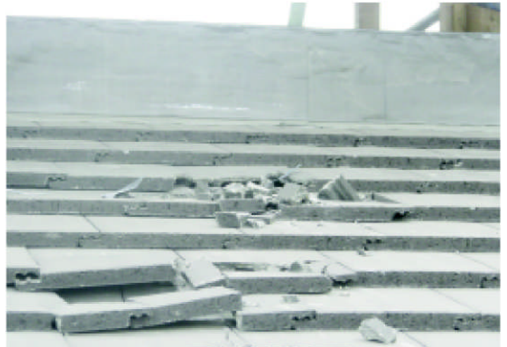
This is the damage left after the scaffolders dropped the scaffold.
