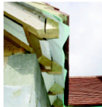
The roof was completely tiled with clay plain tiles before the carpenter had finished the rafter feet and installed the fascia boards.
