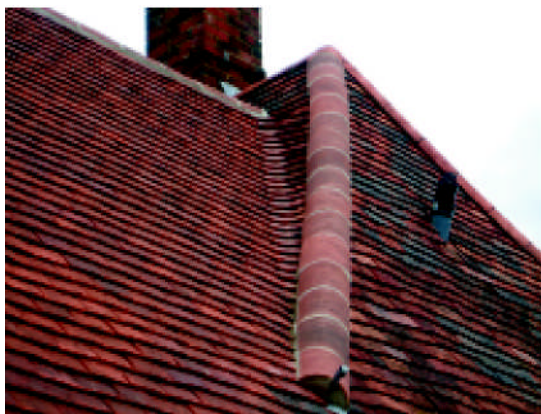
Because of the differing rafter pitches, a valley and a hip converging in the middle of a roof. The hip tile at the bottom of the valley is blocking the natural water flow and causing water to back up through the tiles and causing a roof leak.
