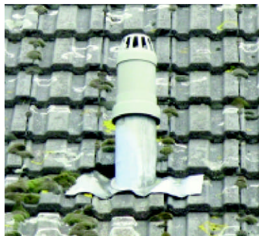
The base sheet on this lead saddle was only 400 x 400 giving approx 100mm of side lap. Notice the pipe has sunk into the roof creating a rat hole under the tiles above. At least the top edge of the lead pipe is protected by a plastic collar.
