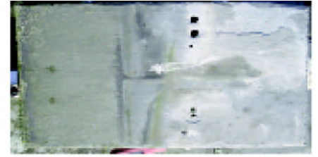
This slate has three sets of nail holes. Only one is the right size, as the slate is soft and flaking, suffering from frost delamination. Note the lines of the side and headlaps of the slate above.
