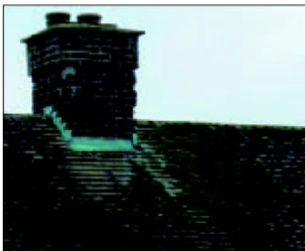
limited area of roof free from moss.
