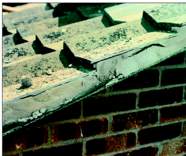
~ The black line running through the mortar is the edge of the underlay, which was soaking up rain water and transferring it into the loft. The underlay should be under the undercloak, not above it. Also these Delta tiles can not be nailed so they should be clipped using verge clips. Where are they?
