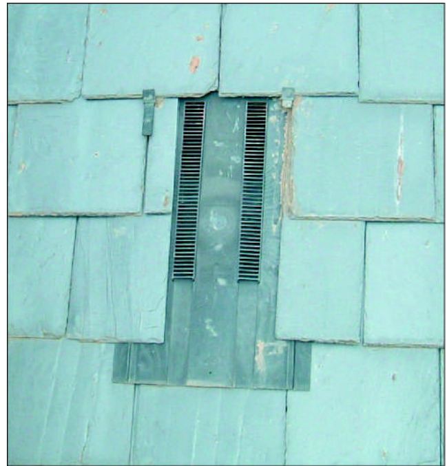
~ This looks nothing like the illustration in the fixing instructions. The slates above are held in with plastic remedial clips, the slates on the side are held in with mastic and the lower ones are too narrow. While at the bottom the vent is laid straight bond and out of alignment, so a tail rivet fixing is impossible. Altogether a bit of a disaster.
