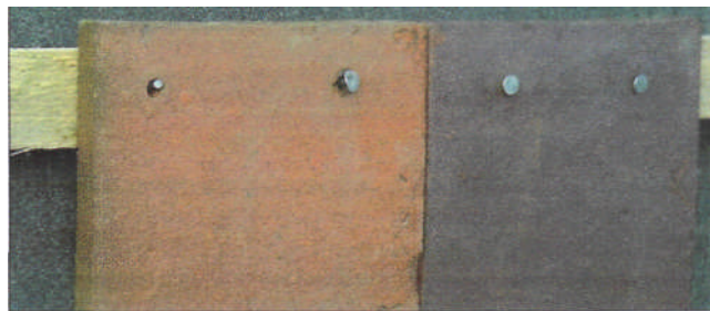
• The heads of 40 by 2.65mm aluminium clout head nails are very thin. Under high wind suction the left hand nail head has pulled off, the middle nail head has started to fold up and the right hand nail is new, but just as thin.
