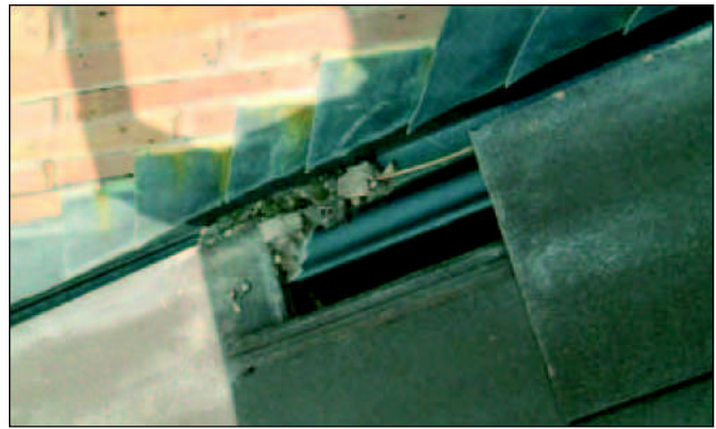
- How not to construct a side abutment. The battens under the GRP secret gutter extend to the face of the wall, kicking it up. This has kicked up the edge tiles making them unstable and difficult to nail into the batten. Note the debris blocking the drainage channel, and the absence of lead cover flashing over the surface of the tiles.
