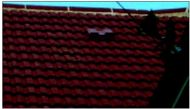
~ One vent tile in a roof slope is not adequate ventilation to comply with either British Standards or Building Regulations. This roof had no low level ventilation, and a vent tile too low to be effective as a high level vent – it should have been installed in the second course below the ridge tiles.
