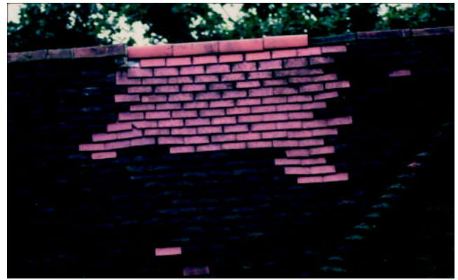
~ Mixing machine-made single camber tiles with hand made double camber tiles is not recommended. Note the tight fit of the hand made tiles, compared to the gaps between the machine made tiles.
