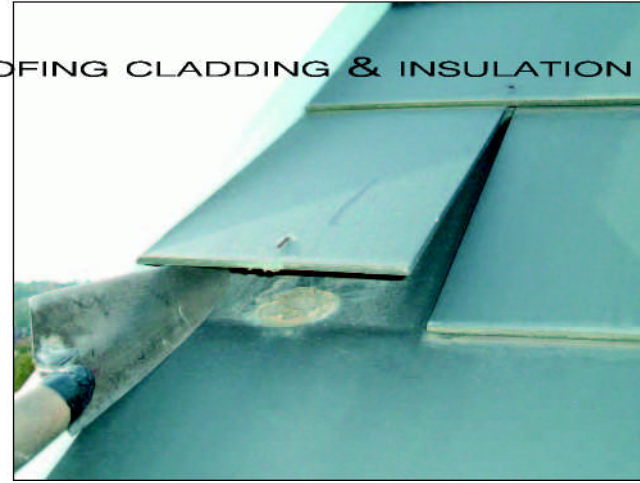
- The use of a half slate at a verge is normally very unstable as it is difficult to get two good centre nail fixings. In this instance, mastic used to hold the slate down failed within 12 months and the copper disc rivet was only fixed to the half slate and not to the slate below.
