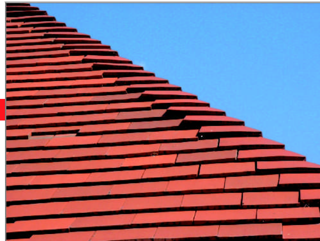
- The clay arris hip tiles on this roof were not sorted correctly. While some of the hip tiles fit correctly, others kick out badly. Note how tile and a half's have been used to maintain the half bond.
