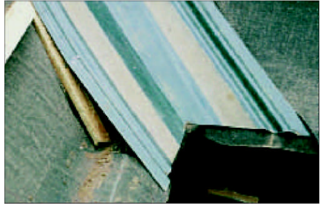
~ This is how NOT to install a GRP valley trough. Note the kink in the GRP at the first nail fixing and how the underlay is dipped behind the fascia caused by the end of the valley batten.
